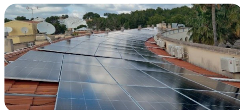
Hotel FLORAMAR Menorca 99,75 kWp
