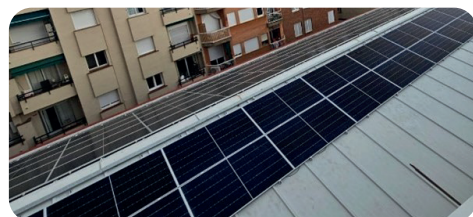
INST. EUROPEO DESIGN Barcelona 126,54 kWp
